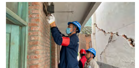
The CDT electric power emergency crew went deep into the earthquake-stricken area. They looked into over 60 km of village lines in seven days and eliminated over 10 hidden dangers, thereby helping over 400 households restore power supply
