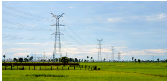
Phnom Penh West – Buddha – Battambang 230kV Power Transmission Project (Cambodia)
