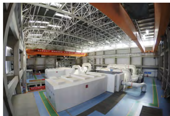
Two sets of units achieved “dual commencement” in cogeneration project of Gaojing Thermal Power Plant of Datang Power in Beijing
